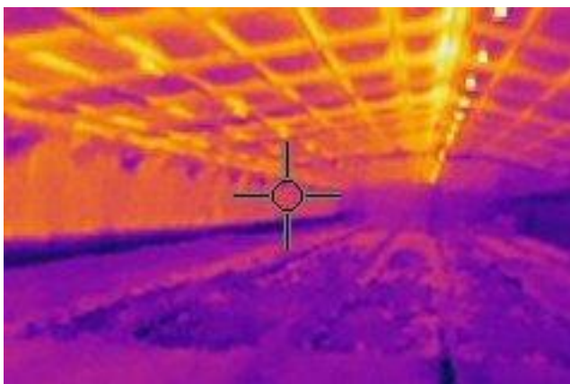
A thermal image shows leakage points (heat entry) in a farm facility. Heat entry can be seen as thermal bridging along the roof beams and through the side walls. Gaps or holes within insulation or in the general building envelope must be sealed to achieve the rated efficiency of your insulation solutions. These types of images are most effective when the temperature differential (deltaT) is greatest between the inside and outside of a building (Image: NSW Farmers 2013, using a FLIR i-7 thermal imaging camera).
